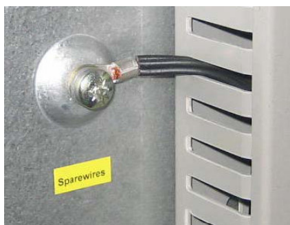
Figure 6.6.1: Earthing of spare wires in LV compartment
